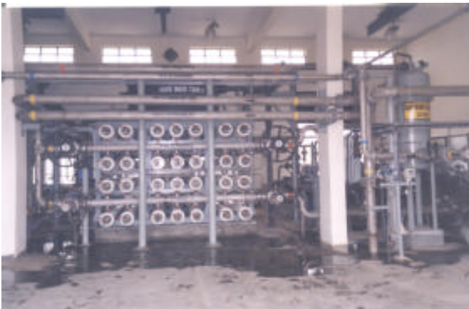
Sea Water Reverse Osmosis (SWRO) Plant building and membrane modules
