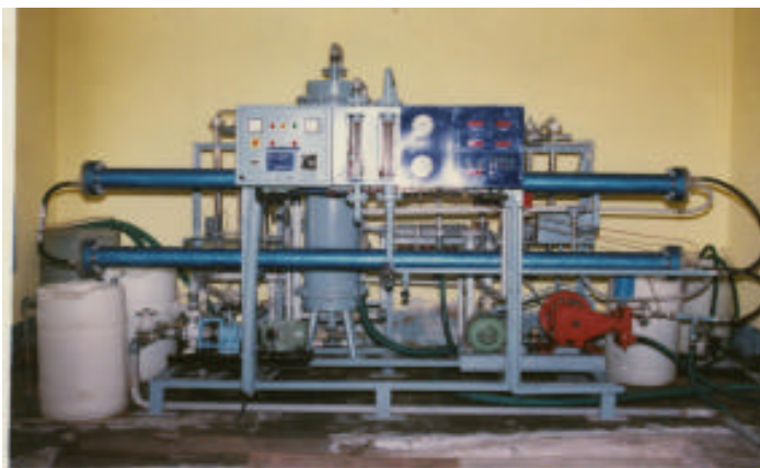
Reverse Osmosis Plant (Capacity : 30 cubic metre per day) set up at Sheelgan village, district Barmer, Rajasthan.
