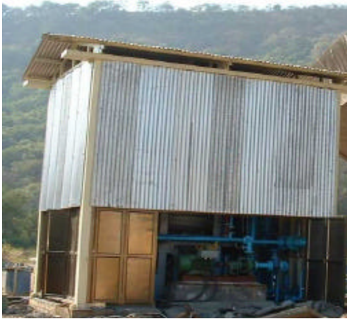
Low Temperature Evaporation Plant at CIRUS
