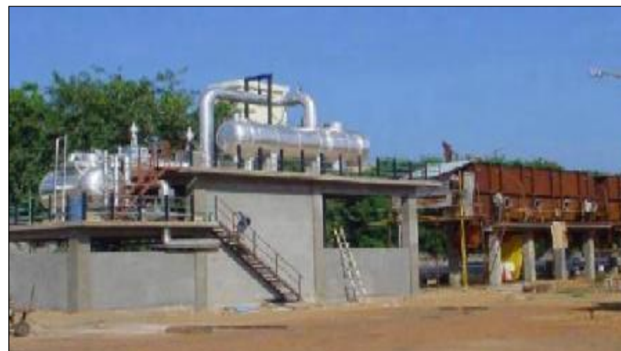
4500 m 3 /day Multi-Stage Flash (MSF) Plant under construction at Nuclear Desalination Demonstration Plant (NDDP), Kalpakkam
