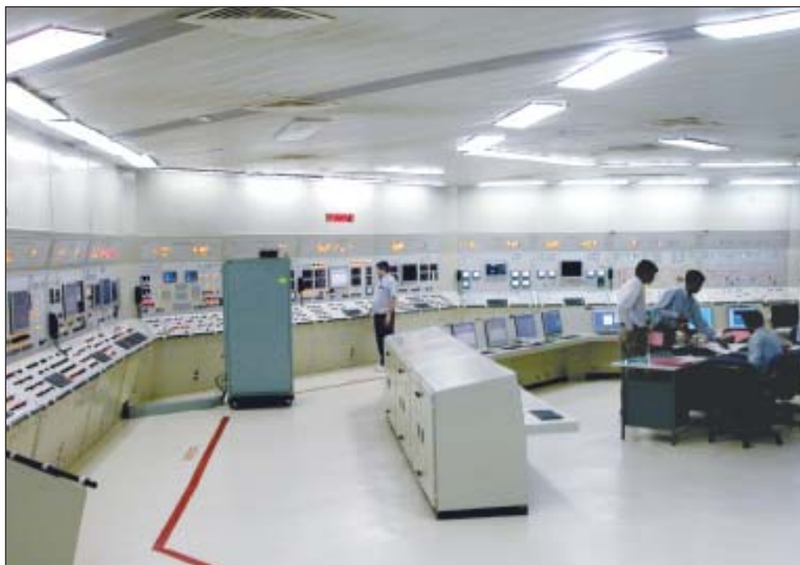
Control Room of Tarapur Atomic Power Station-4
