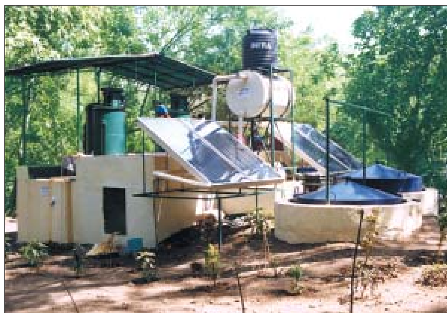
Nisarg-runa Kitchen Waste (Bio-Degradable Waste) Based Bio-Gas Plant
