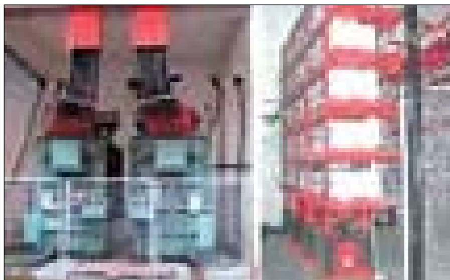
Regulated high voltage power system
