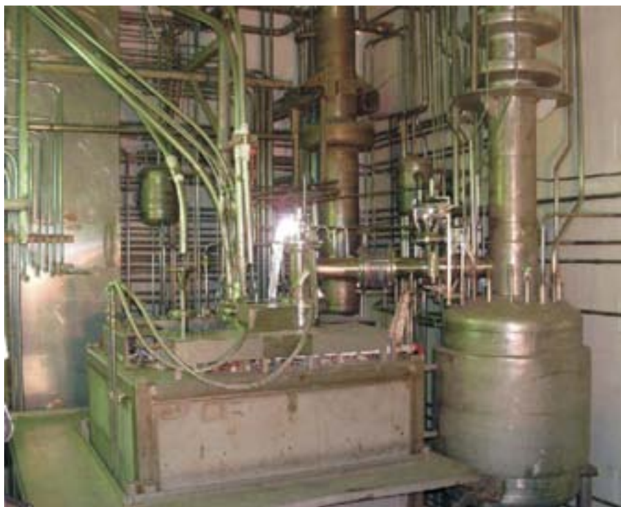
Joule Heated Ceramic Melter at Advanced Vitrification System, Tarapur
