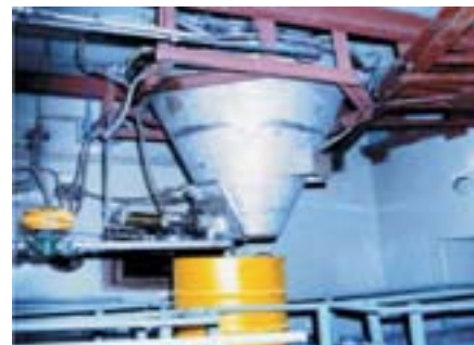
Cementation of sludges using cone mixer assembly at Waste Immobilisation Plant, Trombay
