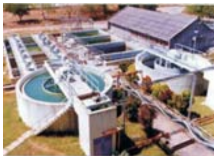
Low level waste treatment by chemical precipitation at Centralised Waste Management Facility, Kalpakkam
