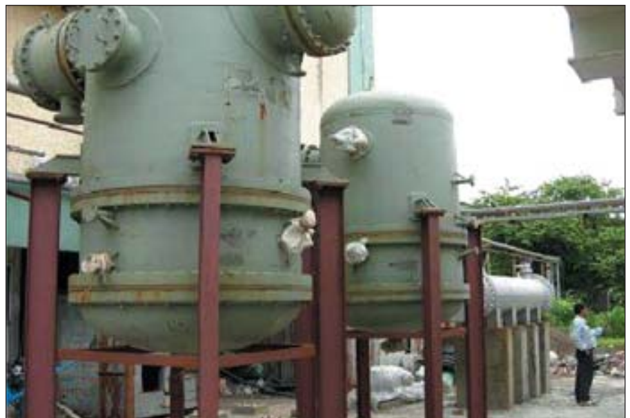
Fig. 2: 50,000 litres/day 2-Effect LTE Desalination Plant (under installation)
