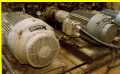
The motors of two hot tower transfer pumps have been made to function as Variable Speed Drive by employing frequency modulator which has helped in saving of power
